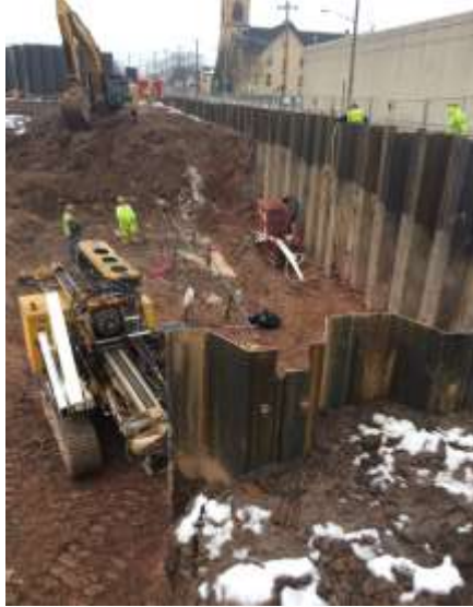
Michels installing the test tieback anchor at the NE corner of the jobsite along Lawrence Street.
