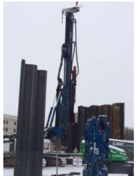
Michels utilizing the diesel hammer attachment to drive sheet piling along the west side of the project.
