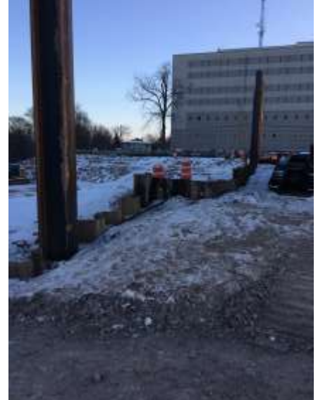
Sheet piling along the west side of the future building driven to depth.
