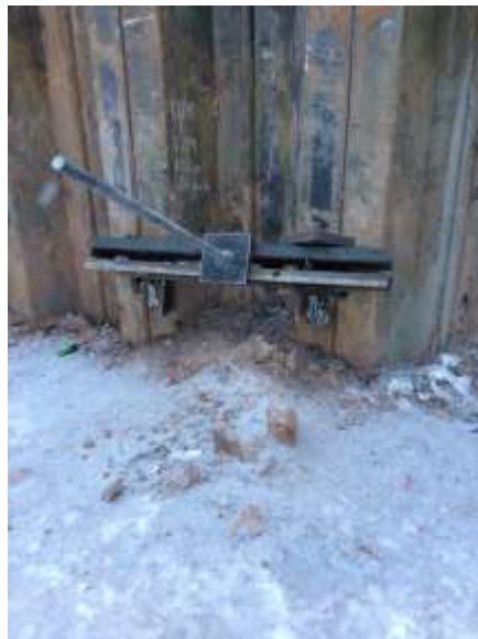
First tieback (test tieback also) completely installed. Rod will be cut back flush with the brace.
