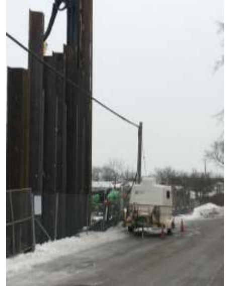
AT&T's temporary fiber splice trailer. This will house the exposed fiber until the sheet piling is completely installed.
