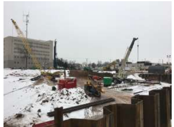
View from the northeast corner of the jobsite that shows the extent of the tier 1 excavation.
