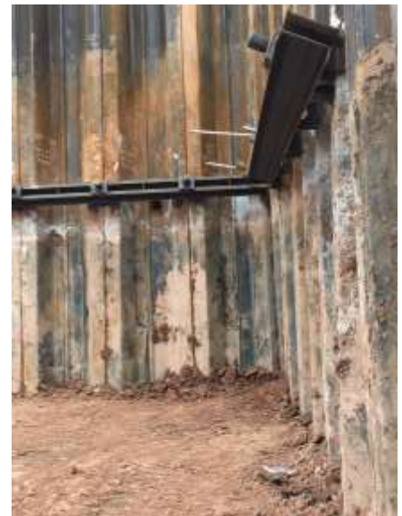
The northwest corner of the project along Lawrence Street shows the depth of Tier 2.
