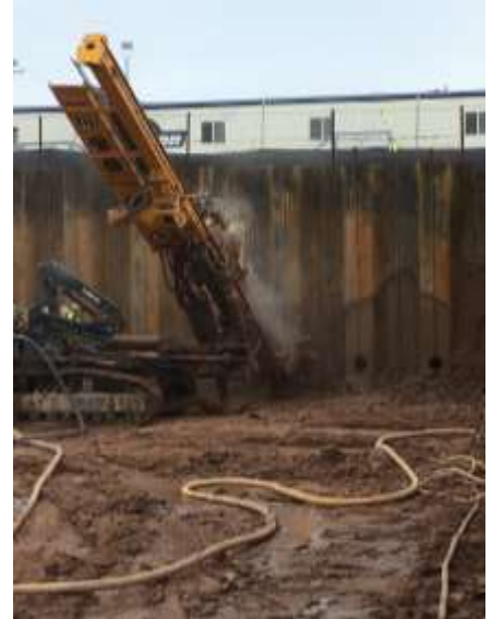
Crews conduct auguring along Elm Street. This picture shows them auguring through abandoned concrete material utilizing a heavier duty coring bit.
