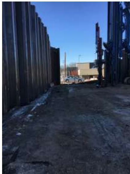
Remaining sheet piling along Elm Street that needs to be driven to depth.
