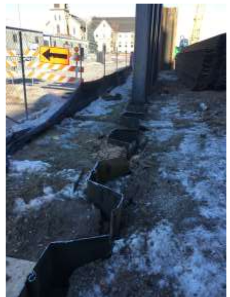
Some of the progress made driving the sheet piling to depth at the corner of Elm and Eighth Street.
