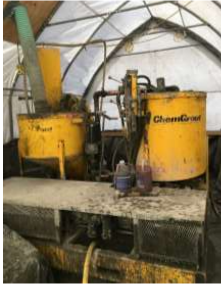
The grout mixing machine located within the temporary enclosures. The grout froze within the hoses approximately 50 feet after leaving the mixer.
