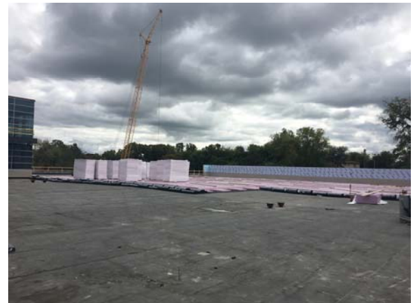
Foam is being installed on the plaza deck, and concrete will begin soon.
