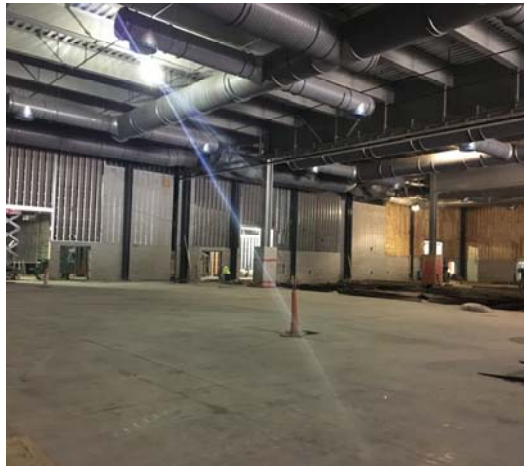
The south third of the exhibition hall floor has been poured. The next concrete floor pour will be the north third of the exhibition hall.
