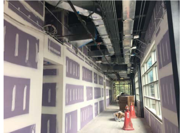
Drywall is being finished in the administration area, and painting has begun. Drywall also continues in back-of-house.
