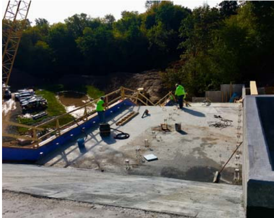
Work continues on the staircase from the park to the plaza deck.
