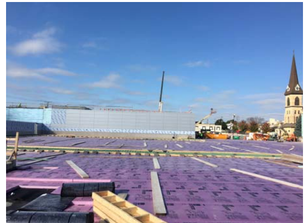
Foam is installed on the plaza deck; forms and tent anchors are in place for the first pour.
