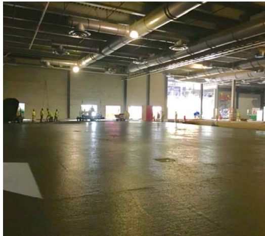
The north third of the exhibition hall floor was poured on Monday, and the middle and final third will be poured Tuesday.
