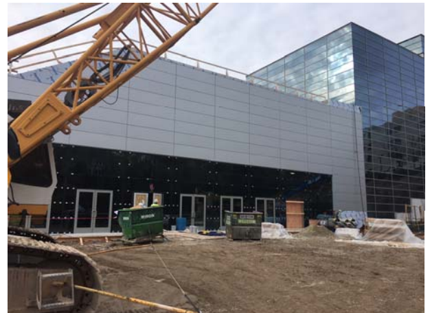
The curtain wall and glazing are complete in the pre-function area leading out to Jones Park.
