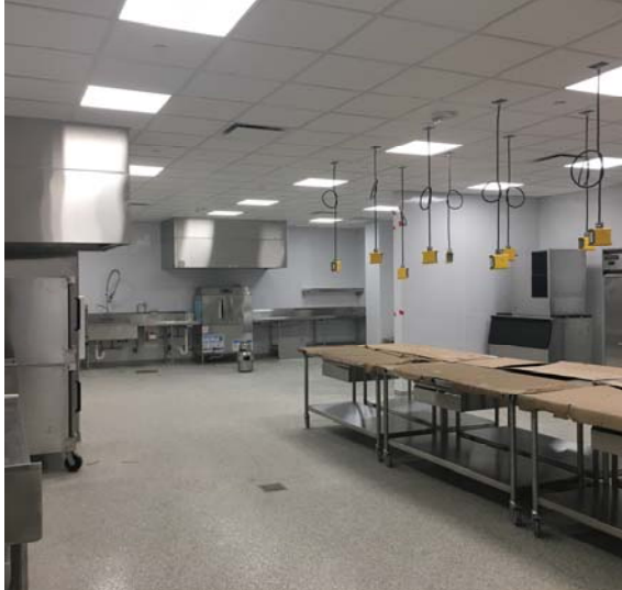
Equipment is installed in the plating kitchen.
