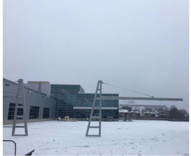
Height restrictors are installed on the plaza deck.
