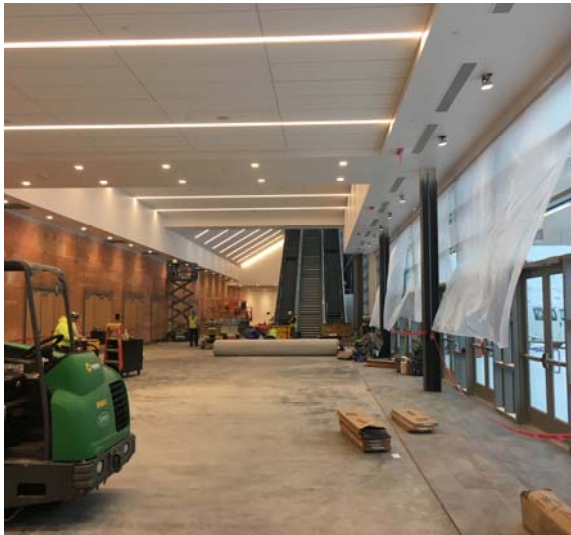
Light fixtures, doors, and tile is installed in the pre-function area. Carpet is ready for installation.
