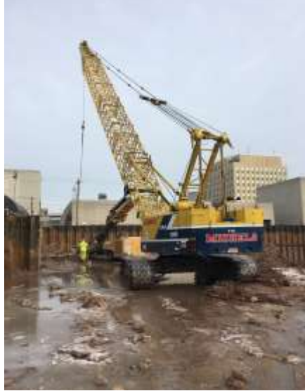
Michels crane hoisting the few remaining tiebacks into the augured out holes along Elm Street.
