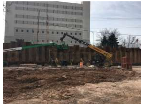
Work continuing on the final grouting of the Tier 1 tiebacks along Eighth Street.
