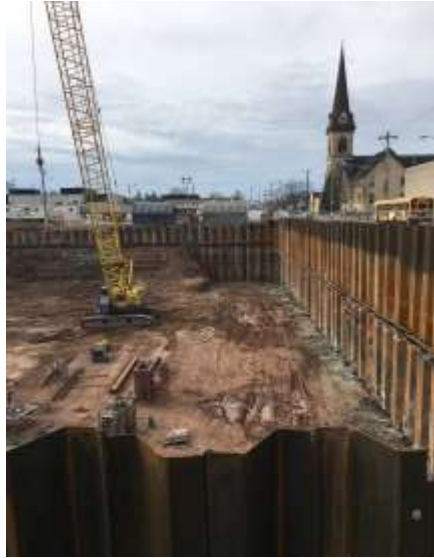
Tier 2 tiebacks have been installed along Lawrence Street, and crews are ready to turn onto Elm Street once the excavation of the soils is complete.
