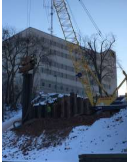
Michels driving the remaining shorter sheet piling into the southeast corner by utilizing the vibrating hammer attachment for the crane.
