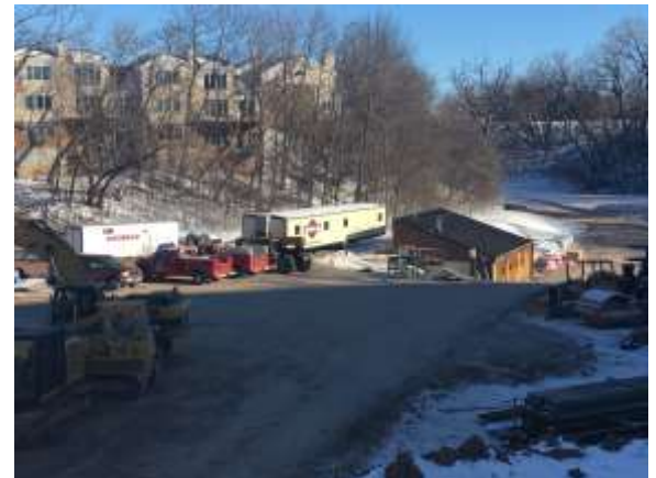
Michels trailer and the Miron concrete trailer being staged next to the warming shelter, which has been converted into a rest/working area.
