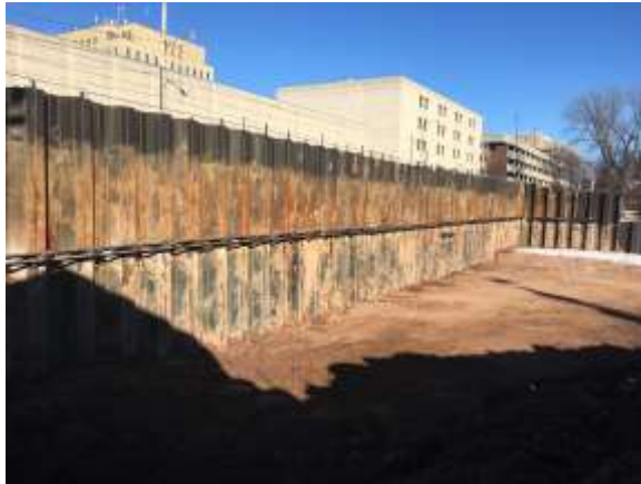
View of the tier 2 excavation progress as seen from the northwest corner of the building limits.
