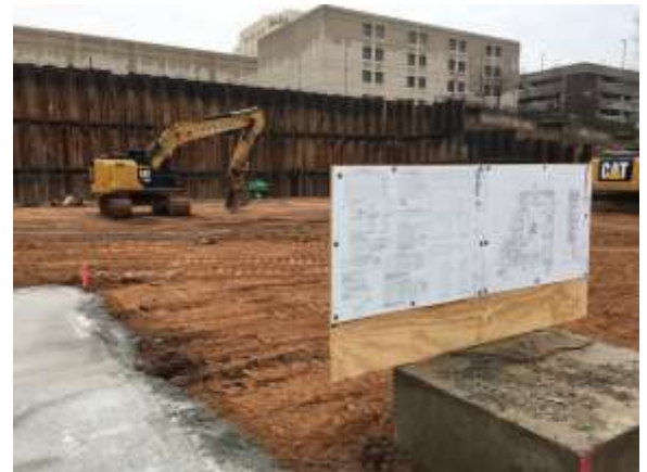
Miron's mud slab being used to piece together forms and rebar. The plans are printed on a waterproof material to allow the crews to quickly reference the drawings as they build.
