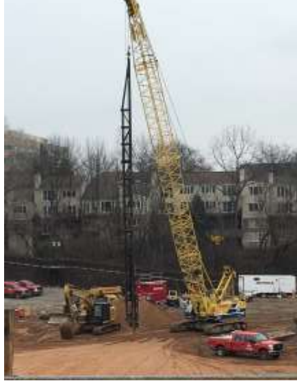
Michels crane with the diesel hammer attachment being staged in preparation for Monday's pipe piling installation.
