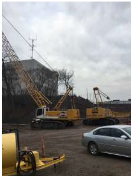
Miron's cranes being erected and staged in preparation for the concrete starting in the coming week.
