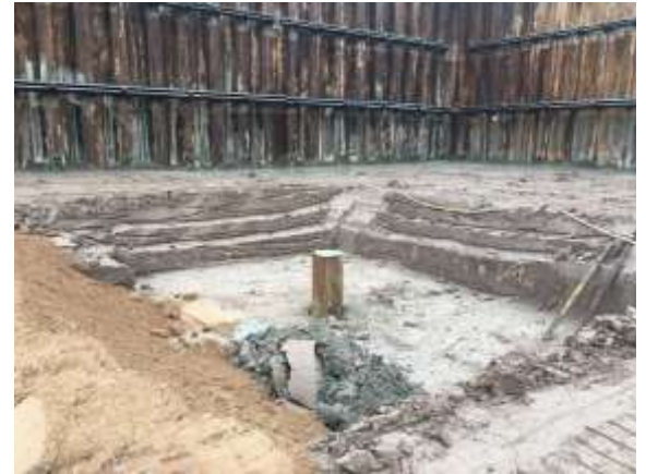
Location of the future freight elevator. The shaft was drilled Monday and the hole backfilled accordingly.
