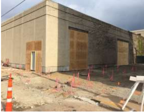
The precast openings have been cut and a temporary enclosure is in place at the Radisson Paper Valley Hotel. Underground utility work has begun.
