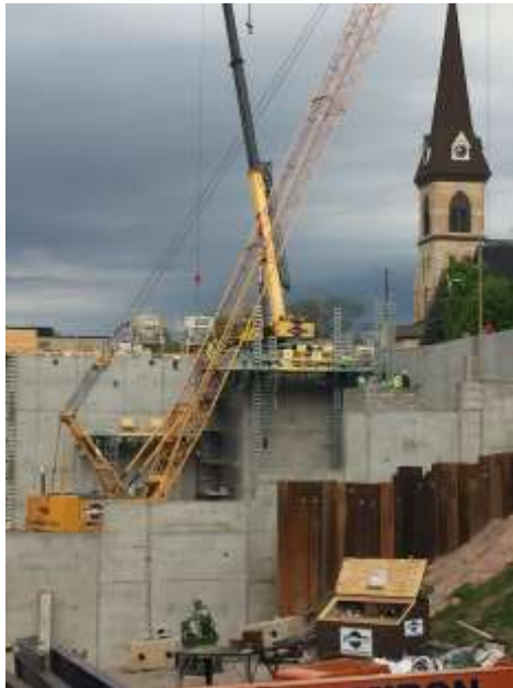
Work started on the northwest elevator shaft earlier in the week and is ongoing.
