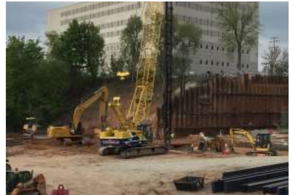
The driving of pipe piles was 100% complete on Friday. Lagging is also complete.
