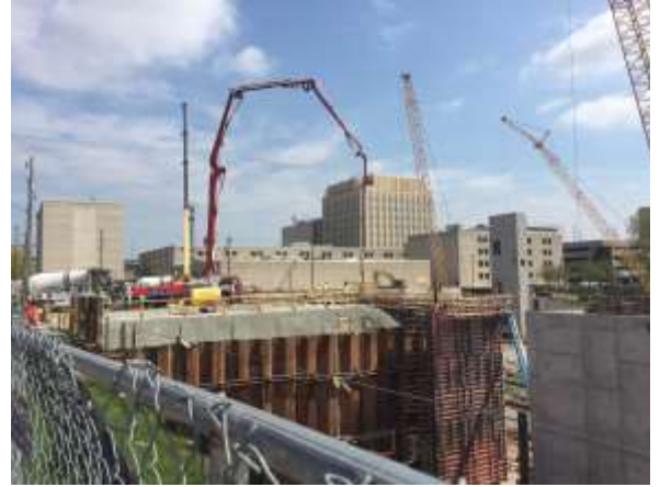
Continuing to form and pour concrete walls along the west side of the project.
