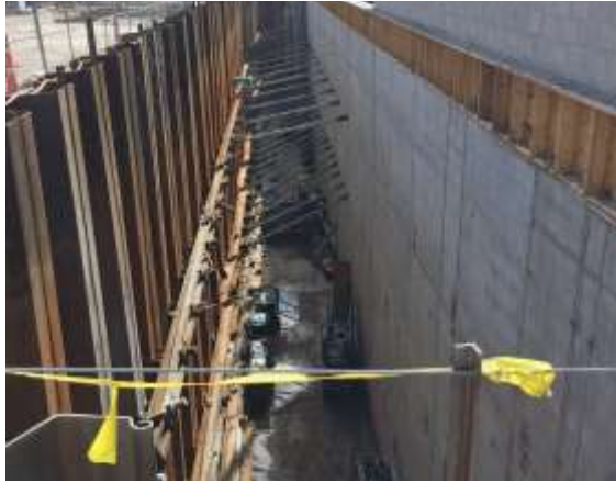
Tieback work between the north foundation wall and West Lawrence Street continues.
