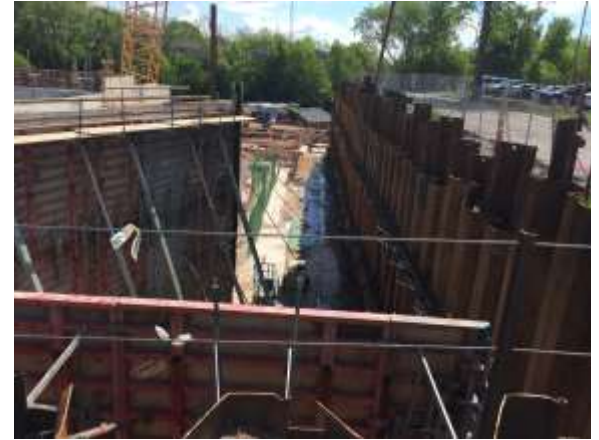
The south wall is beginning to take shape and will be poured later this week.
