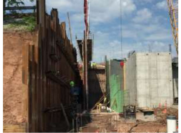
The southwest corner and part of the south wall were poured on 5/26. Work will continue on the south wall.
