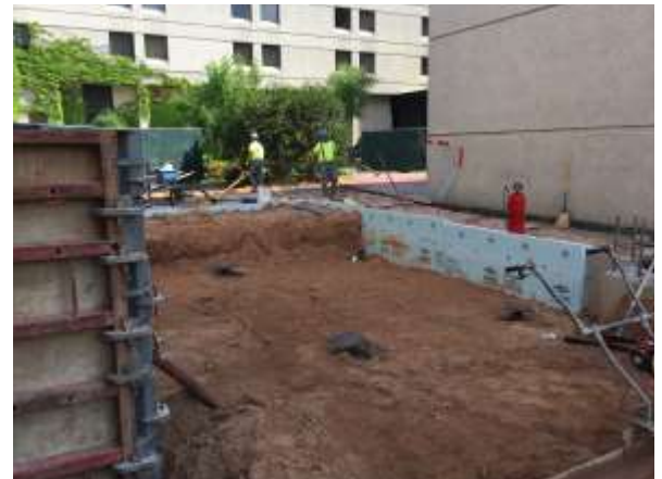
Several helical piles are in place and a new concrete pad is complete in the patio area.
