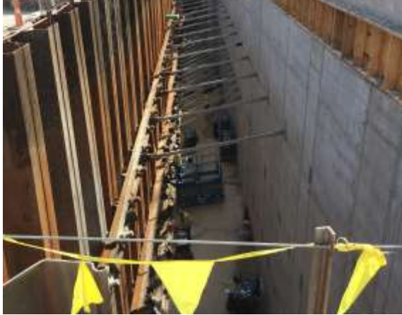
Tieback work between the north foundation wall and West Lawrence Street is continuing.
