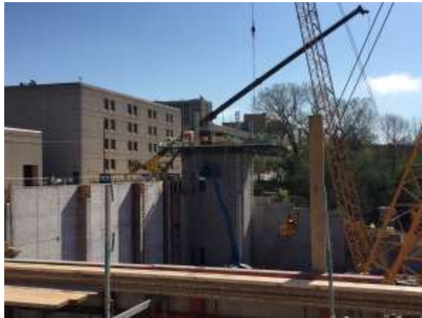
The elevator shaft in the northeast corner of the project is almost complete.
