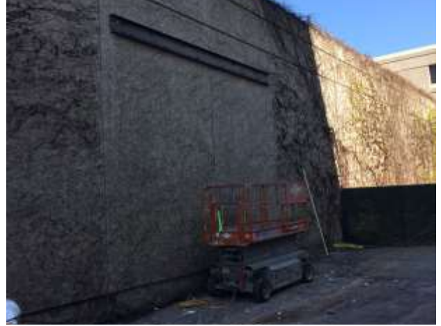
Crews preparing to cut a hole in a precast wall that is located in the alley/courtyard of the Radisson Paper Valley Hotel.
