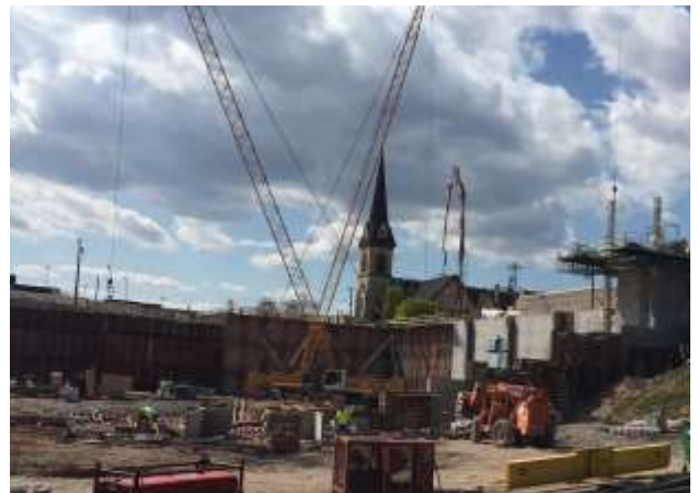
Poured concrete foundation walls are complete next to west Lawrence Street. Crews are starting to form and pour along the west side.
