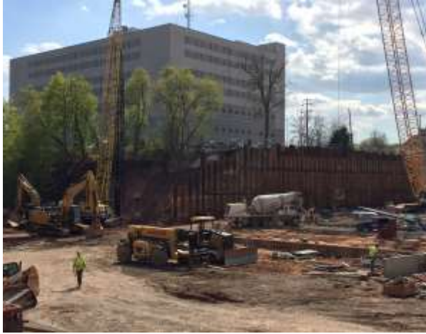
Tieback work on the south side of the project is almost complete.
