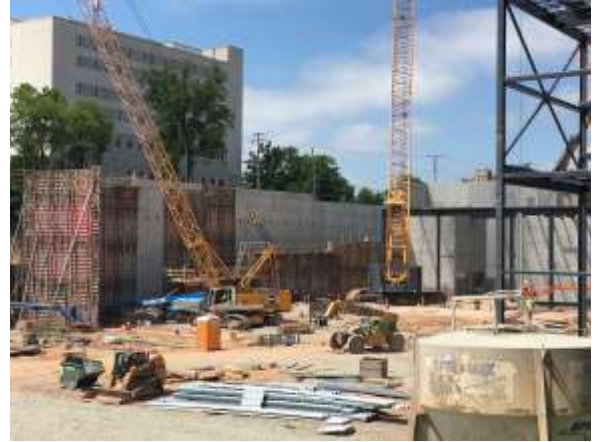
Work continues on the south foundation wall, establishing the southeast corner formwork.
