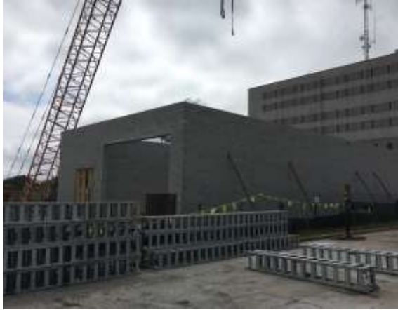
CMU walls are built in the loading dock/service area on the corner of Elm and Eighth Street.
