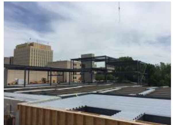
Steel decking is being installed in preparation for a deck pour at the loading dock area.
