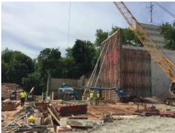
Concrete pours have turned the corner along the southeast wall and will continue along the east wall.
