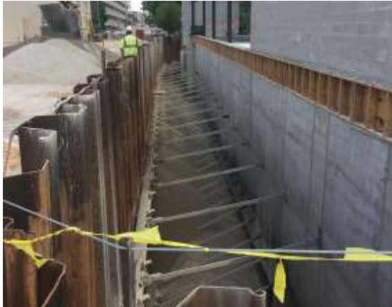
Backfilling along West Lawrence Street and the north foundation wall of FCEC.
