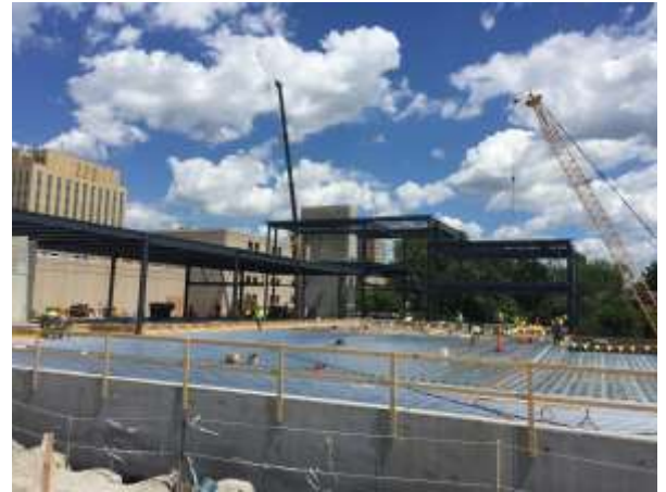
Steel decking installation at plaza level. Carpenters are installing wood forms in preparation for the deck pour at back of house.
