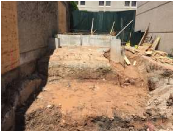
Helical piles have been installed for footings to be formed and poured in preparation for the escalator install.
