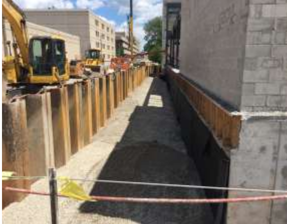
Backfilling along West Lawrence Street and the north foundation wall of FCEC continues.
