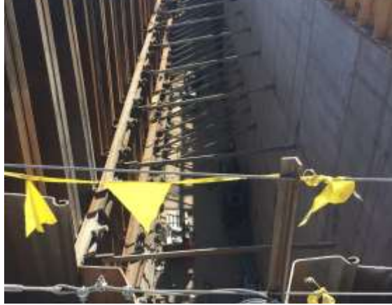
Tieback work between the north foundation wall and West Lawrence Street is almost complete.
