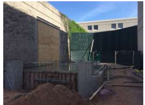
Concrete footing/foundation work continues at the Radisson for the future escalator that will connect up to the walkway over West Lawrence Street.
