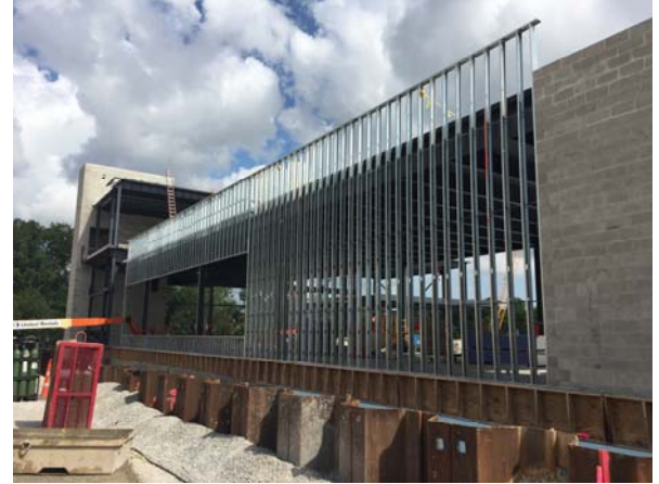
Metal stud installation began this week along the north wall of FCEC.
