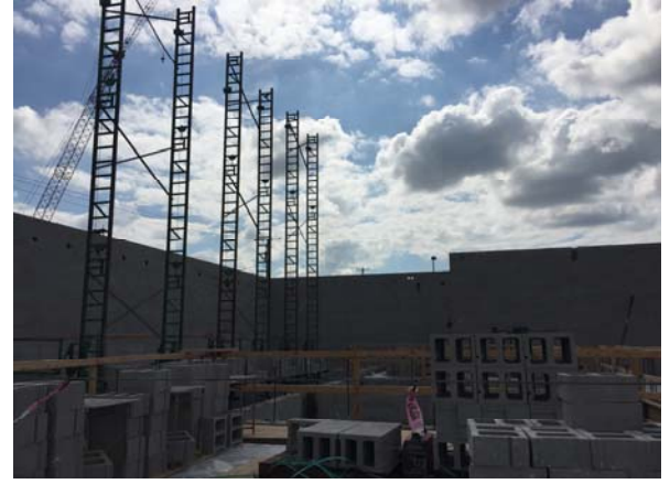
Masons have mobilized to start work at freight elevators and loading dock area.
