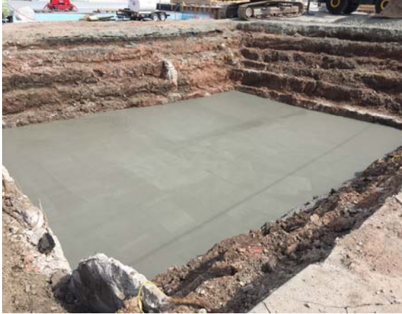
A concrete slab was poured for future installation of a storm water trap tank.
