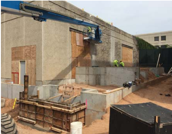
At RPVH: Foundation work is wrapping up and backfilling is taking place as needed.
