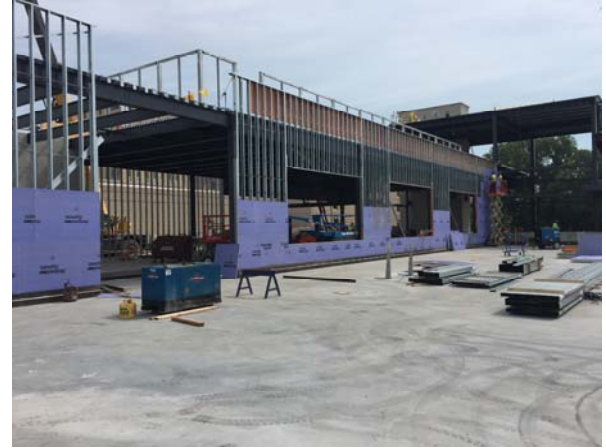
Exterior metal stud installation continues along with installation of exterior sheathing for the administration walls.
