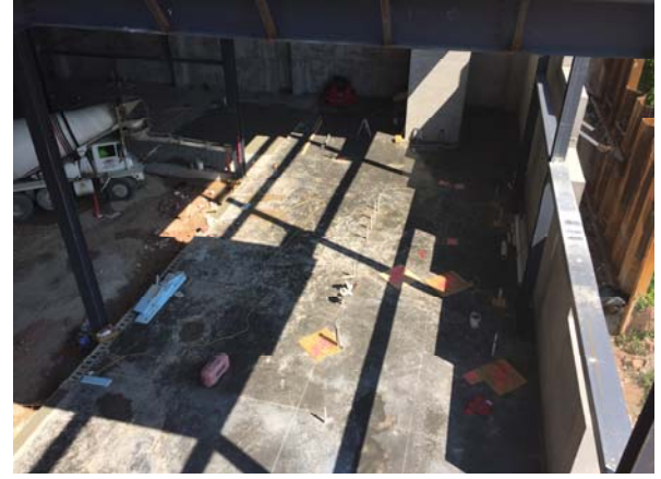
The north portion of the pre-function slab on grade has been poured.
