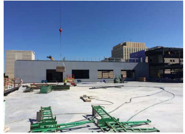
The walls for the administrative area located on the south side of West Lawrence Street have received an air/vapor barrier spray application.
