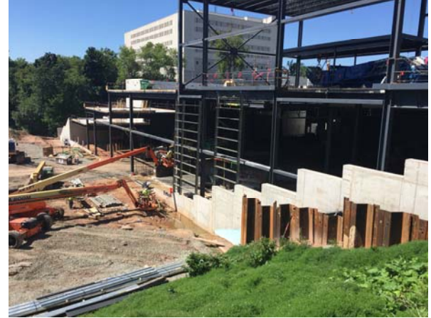
Aluminum curtain wall frame installation has begun on the east side of the exhibition center.
