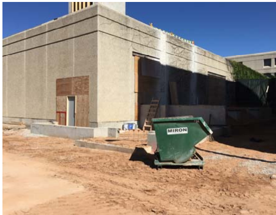
At RPVH: Backfilling is complete. Existing precast walls are prepped for new connections.
