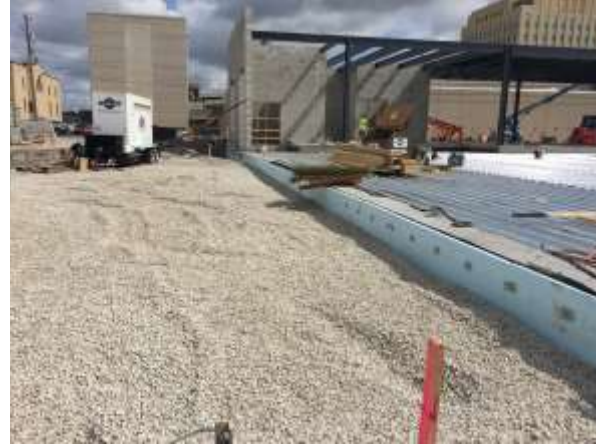
Backfilling along the west side of FCEC is almost complete. Backfilling to continue around the loading dock and south side of FCEC.
