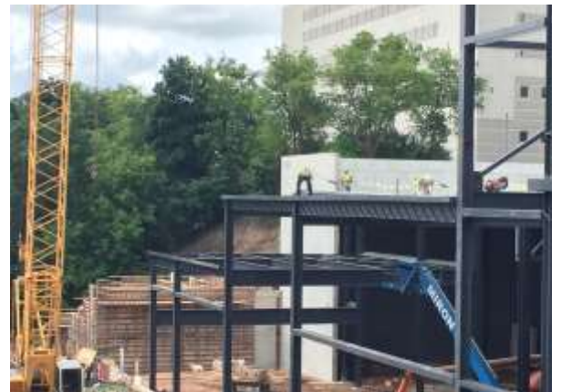
Steel decking at plaza level is being finalized in preparation for upcoming deck pours.
