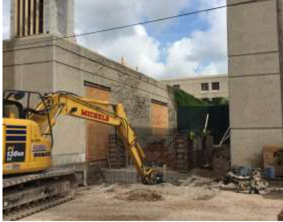
At RPVH: Michels installing helical piles and Miron finalizing the elevator shaft.
